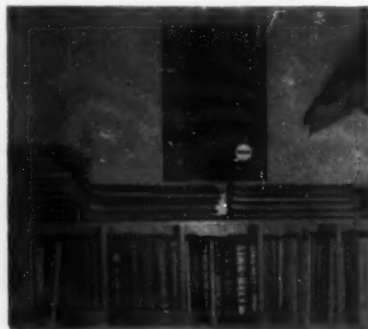
INFORMATION panel shows current activity status of mill equipment.
